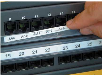
Punch block & patch panel labels
