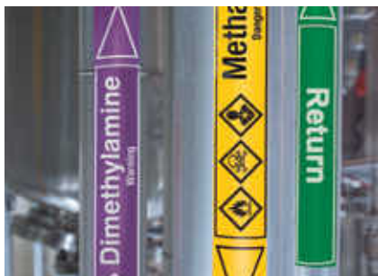
Pipe & valve marking
