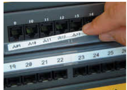
Punch block & patch panel labels
