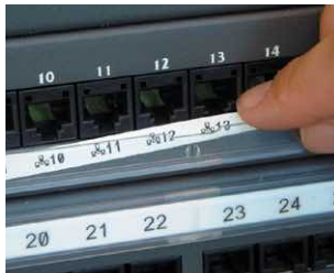
Punch block & patch panel labels
