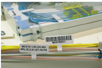
Fibre optic cable markers
