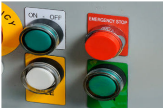
Control panel labels
