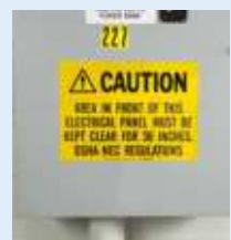
Hazard warning signs
